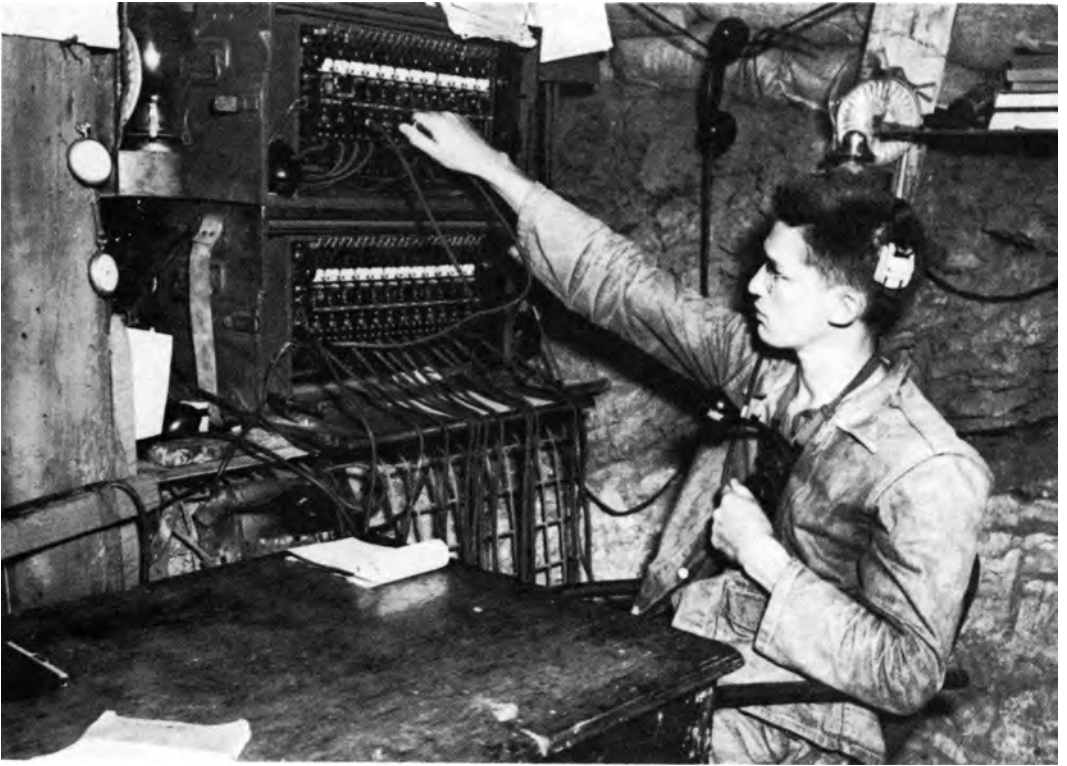
A TWELVE-DROP SWITCHBOARD, the BD-72 , in a communications dugout. ( Photograph taken in 1943. )
